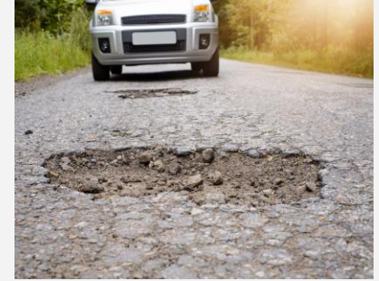
3 Bn$ annual cost of potholes in the US.
